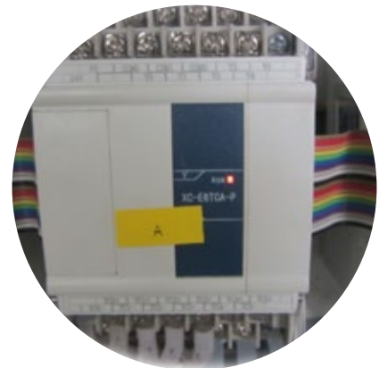
PLC (Made In Taiwan)
